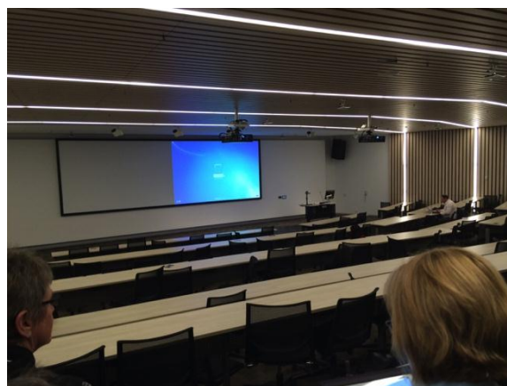
Lecturer theatre at UTS with numerous Wi-Fi access points
