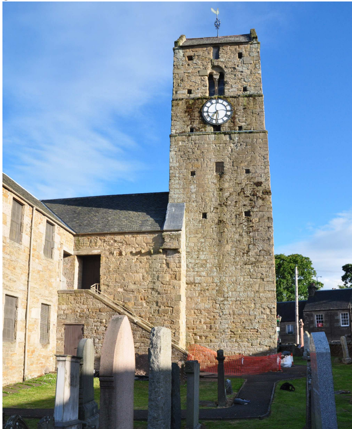
Fig 1 Location of excavation at base of tower with its Romanesque belfrey opening and holes for wooden gallery. Note the 19th-century loft stairway concealing the 12th-century north doorway.
