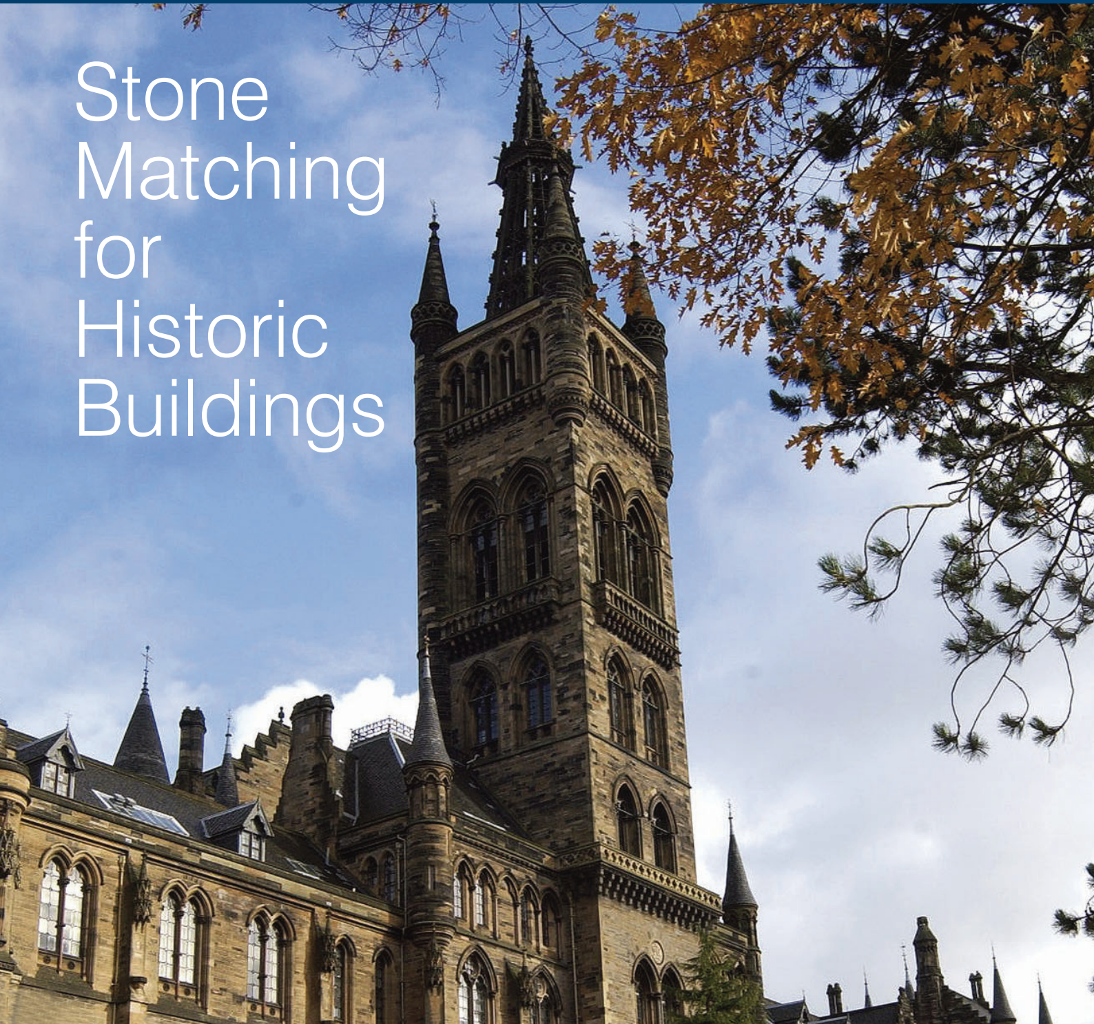
Tower, University of Glasgow – highlighting both decayed and replaced stones
