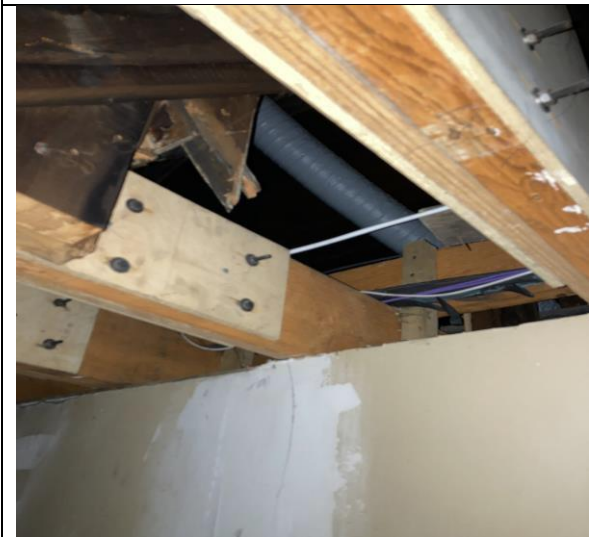
Area (void on L4) for potential fire spread.
