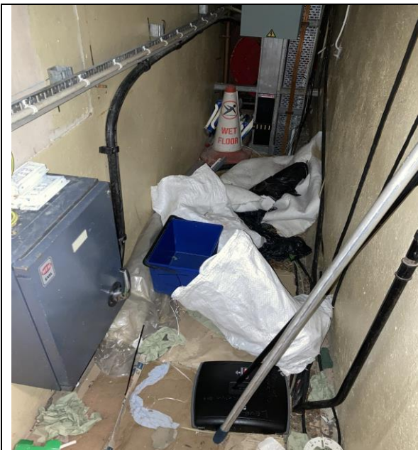
Combustibles stored next to electrical installation.
