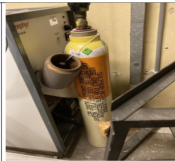
Compressed gas cylinder left in cupboard.
