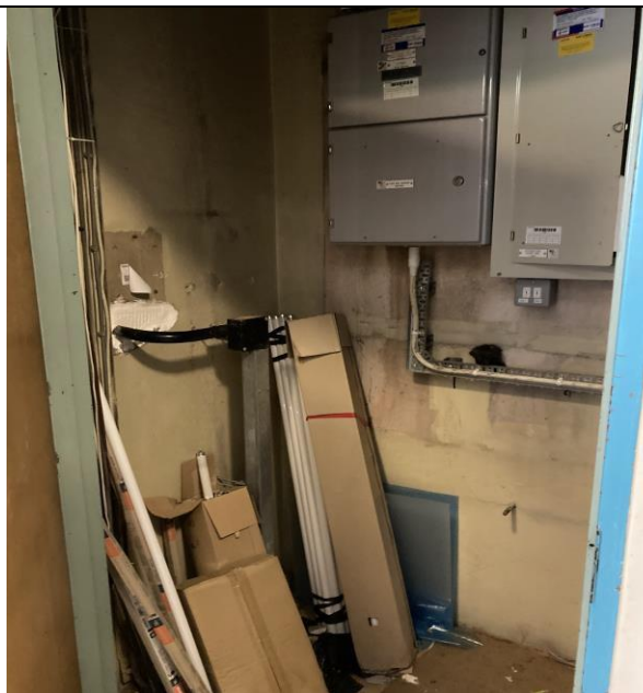
Combustibles stored next to electrical installation.
