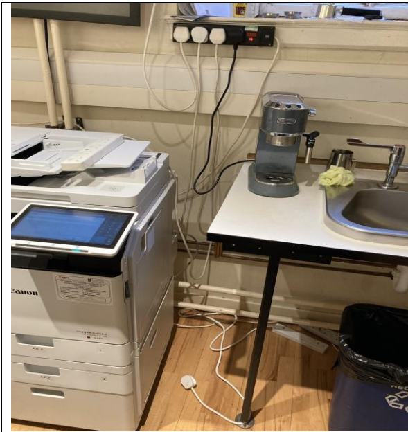
Evidence of daisy chaining.
