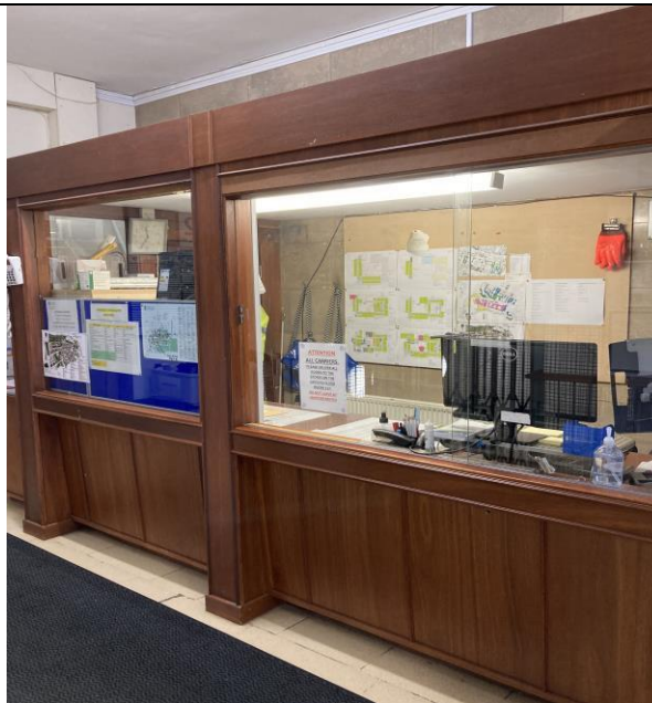
This room requires to be separated from the escape stair by fire resistant material or removed.
