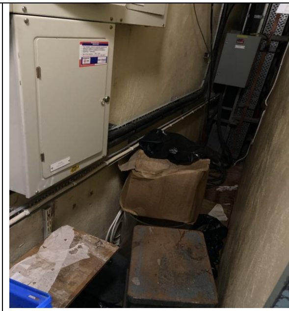
Combustibles stored next to electrical installation.
